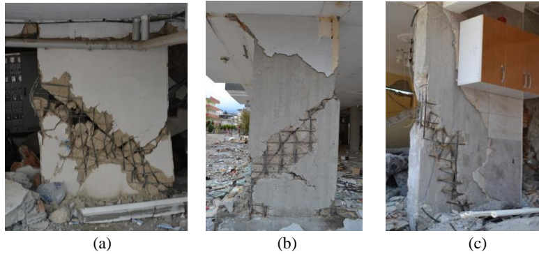
Figure 2a. Examples of reinforced concrete shear walls damaged after 2023 Kahramanmaraş Earthquake Doublet; (Oztürk et al. (2023).
